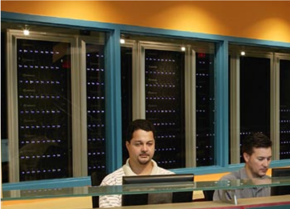
ClearCube PC Blades securely centralized and managed
