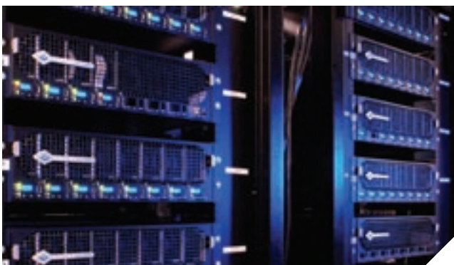
PC Blades secured in data centre.
